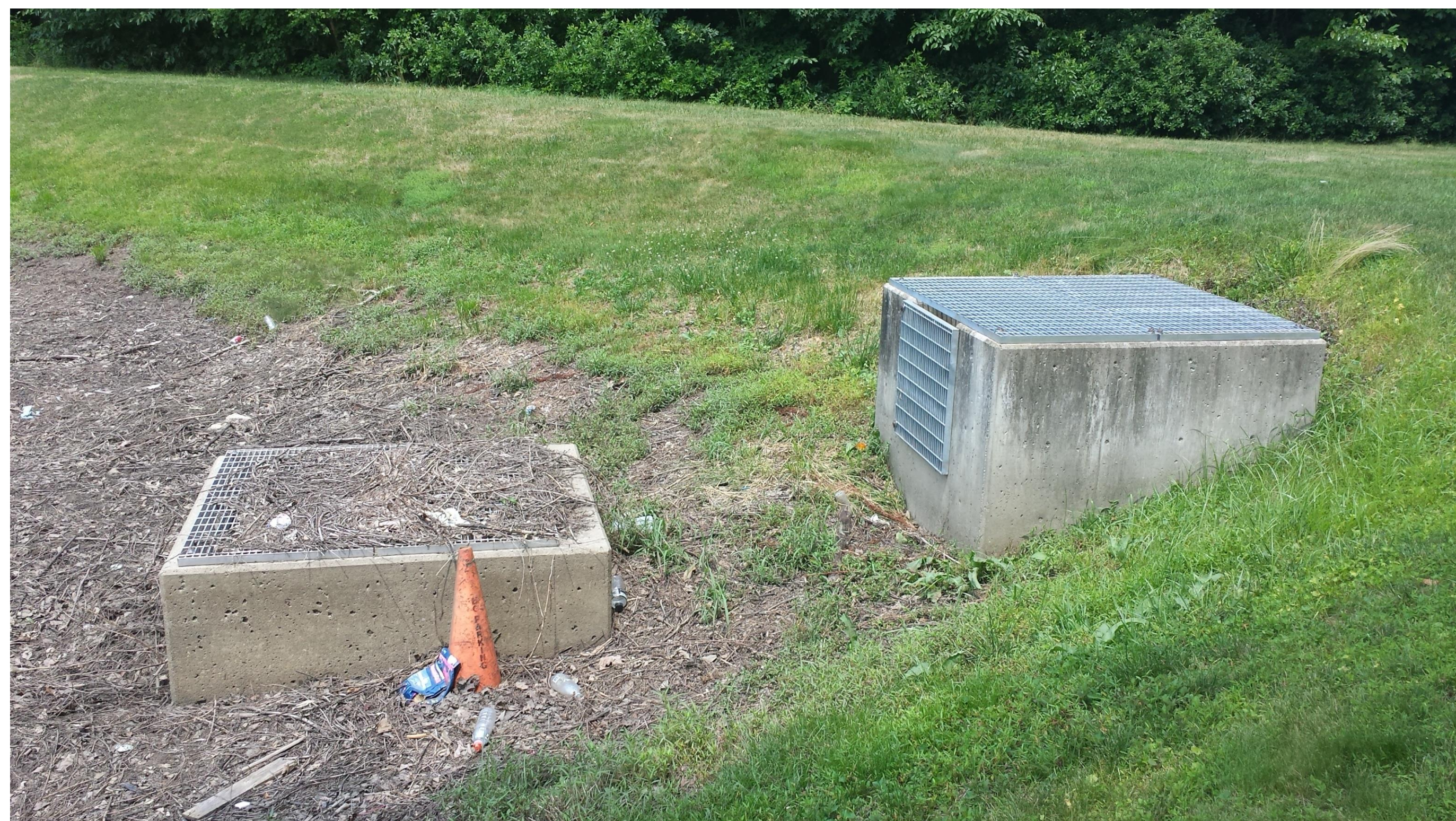
Side view of outlet
