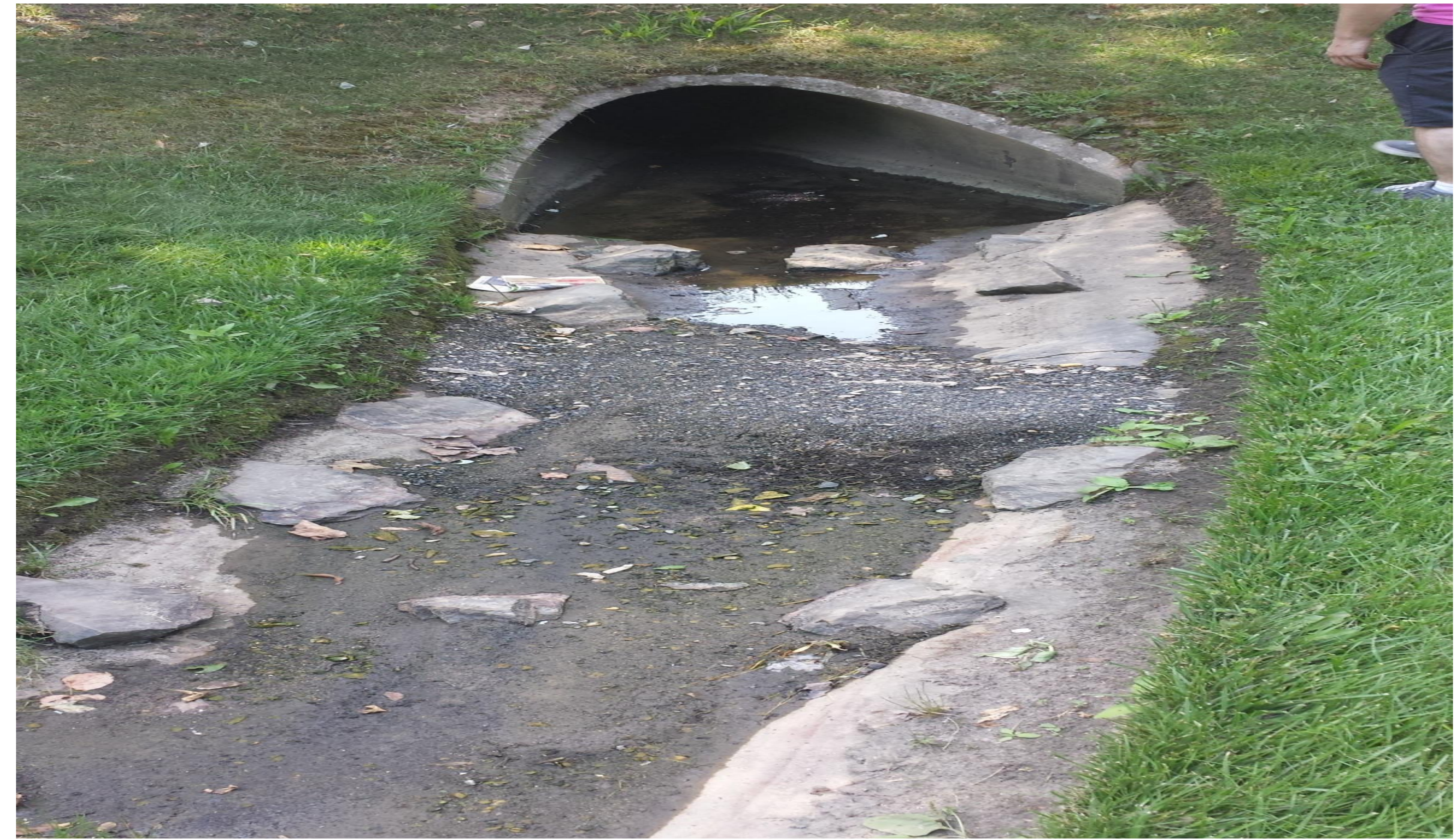
Sediment in low flow channel
