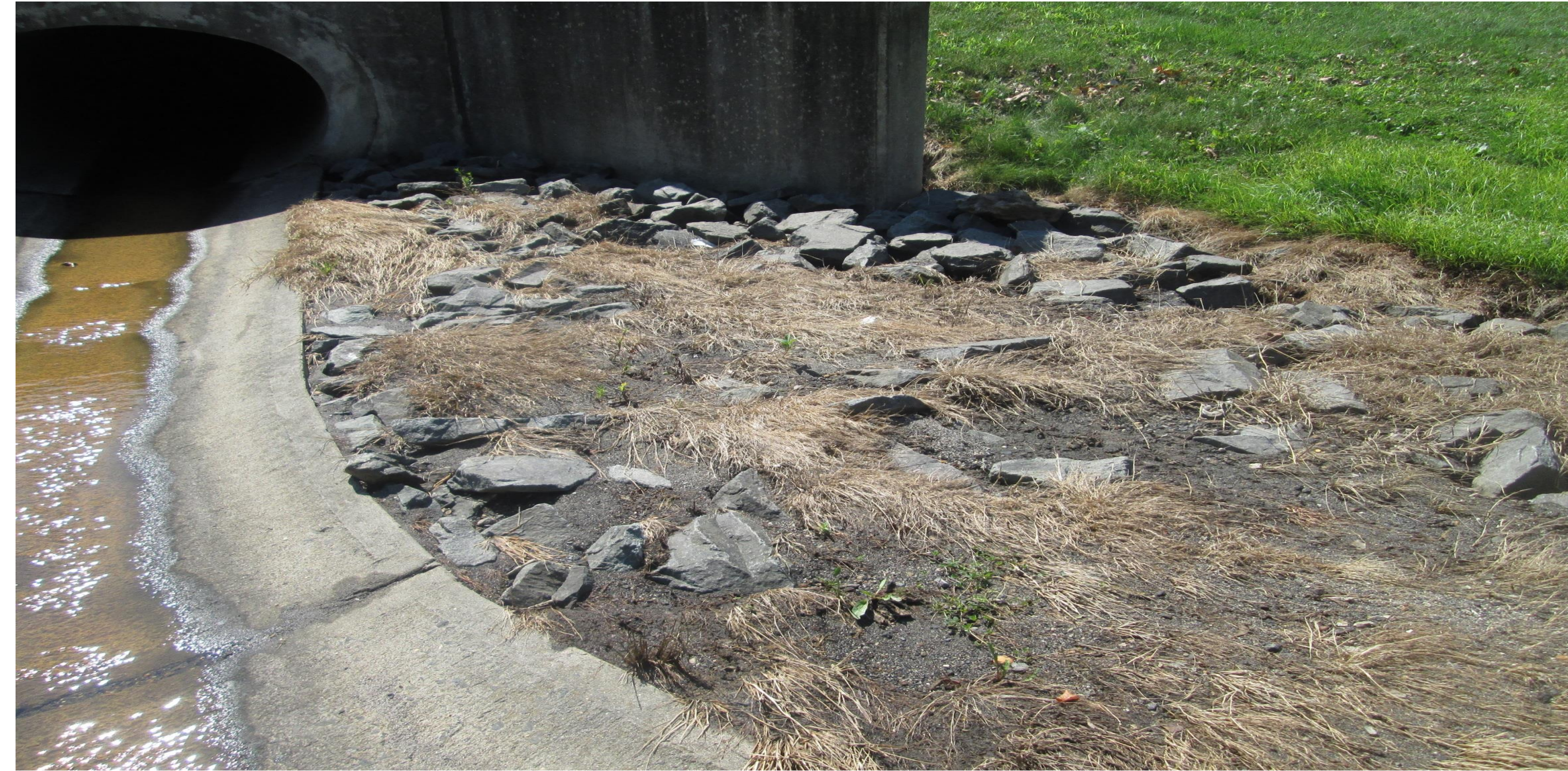
Overgrown rip-rap near inlet
