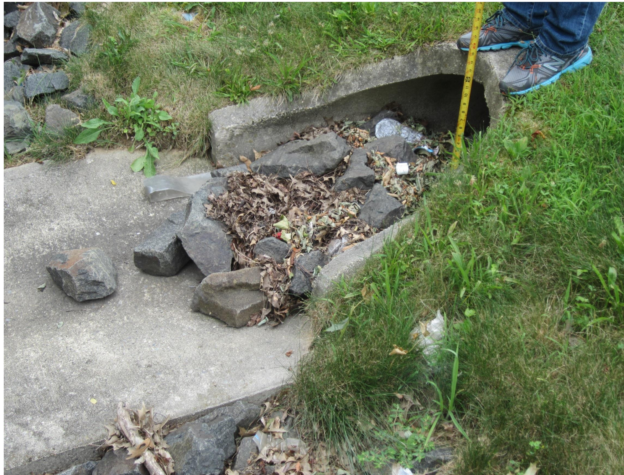
Rip rap, debris, and leaves are restricting the flow of water in inlet
