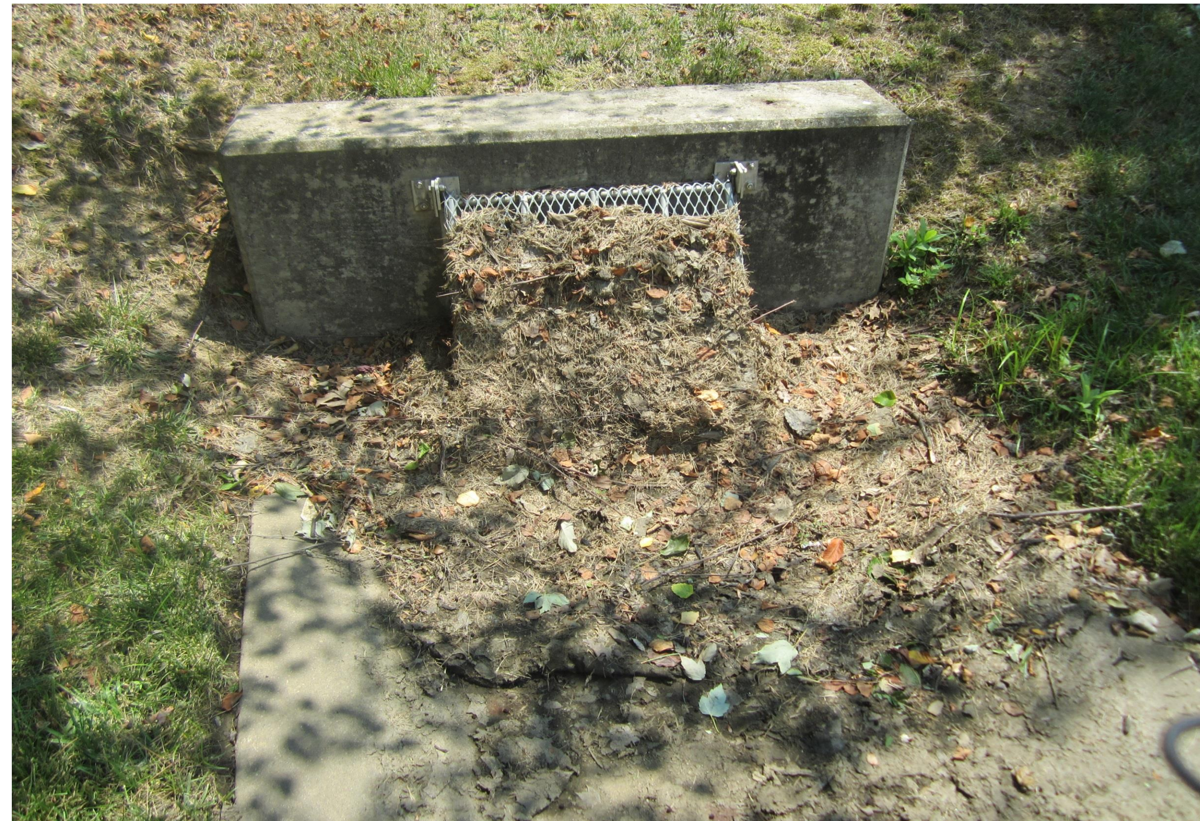
Front view of trash rack
