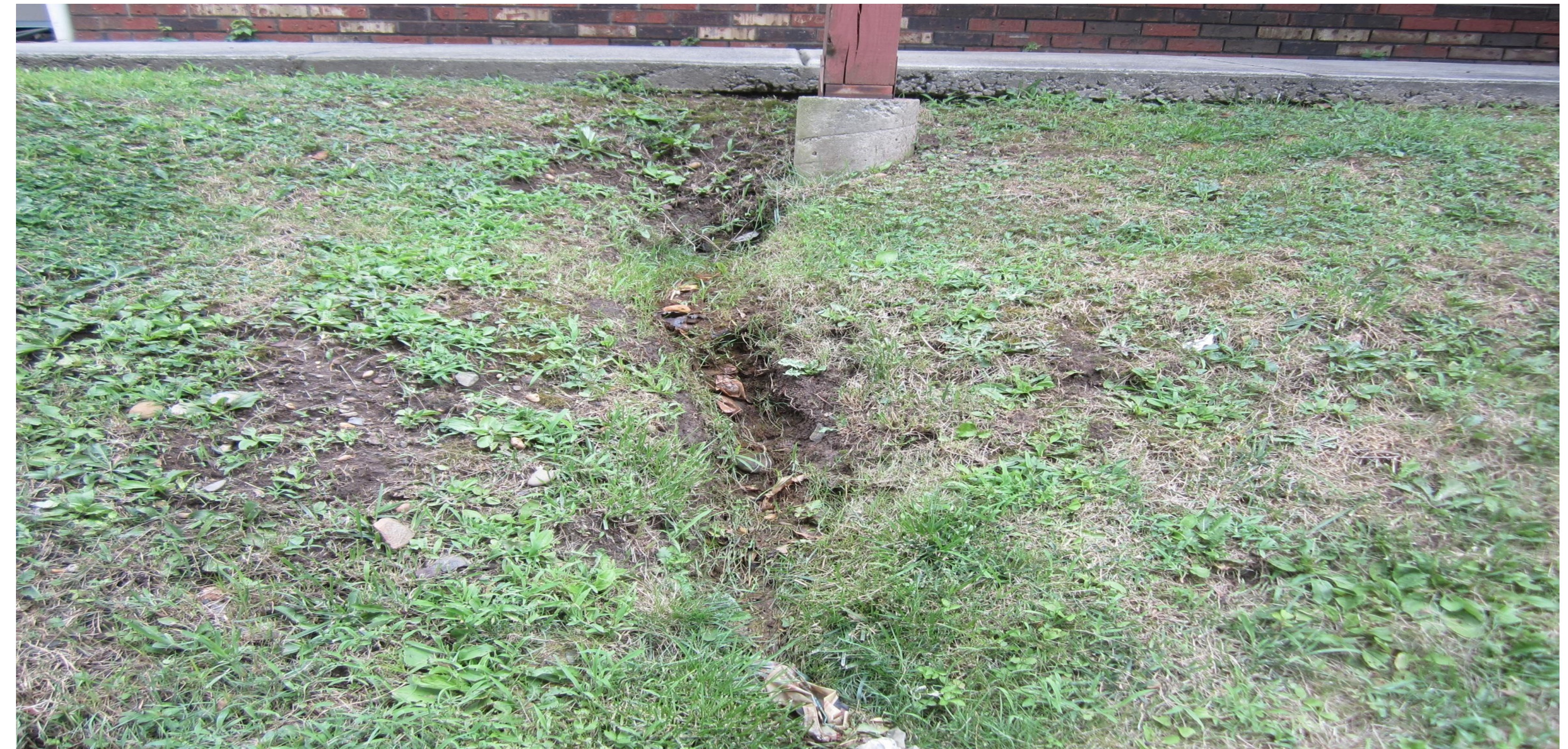
Erosion near eastern embankment
