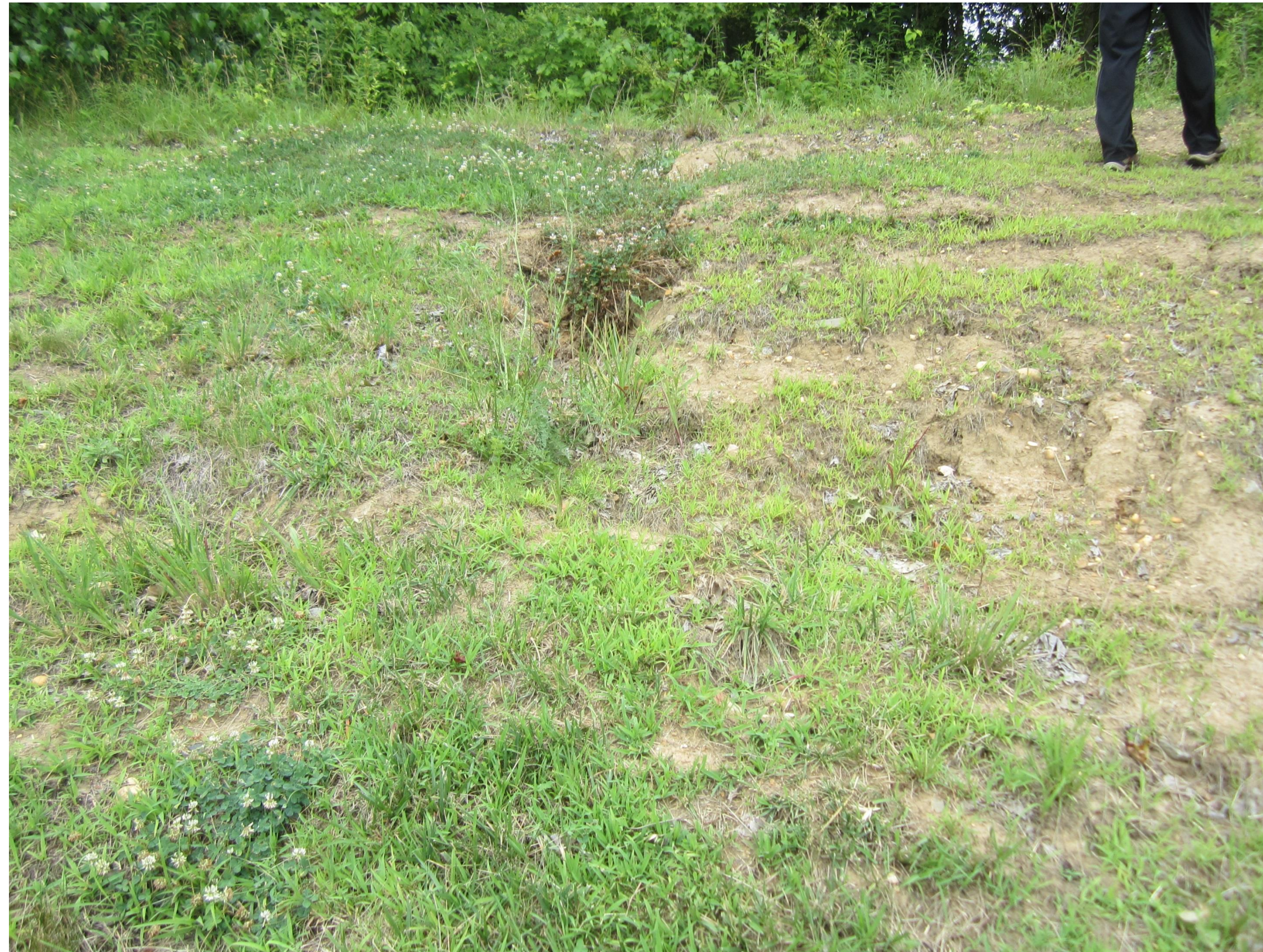
Gullying near west end of swale
