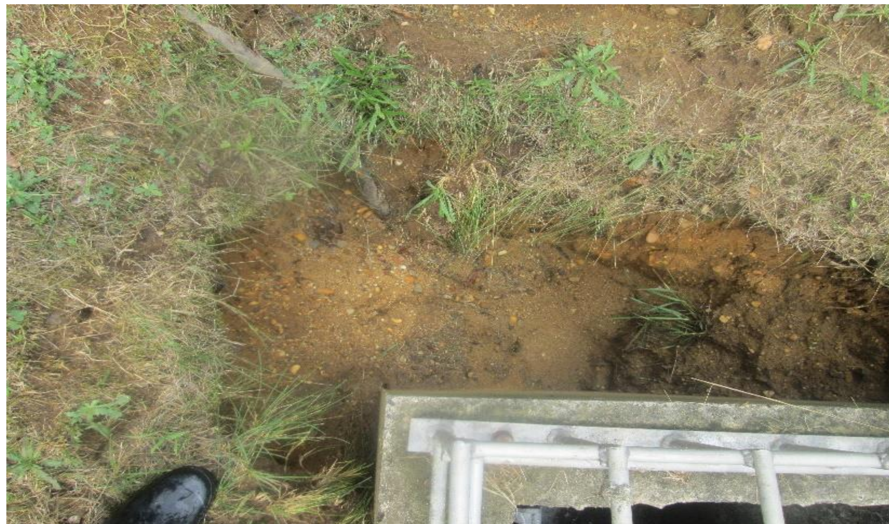
Erosion near outlet structure
