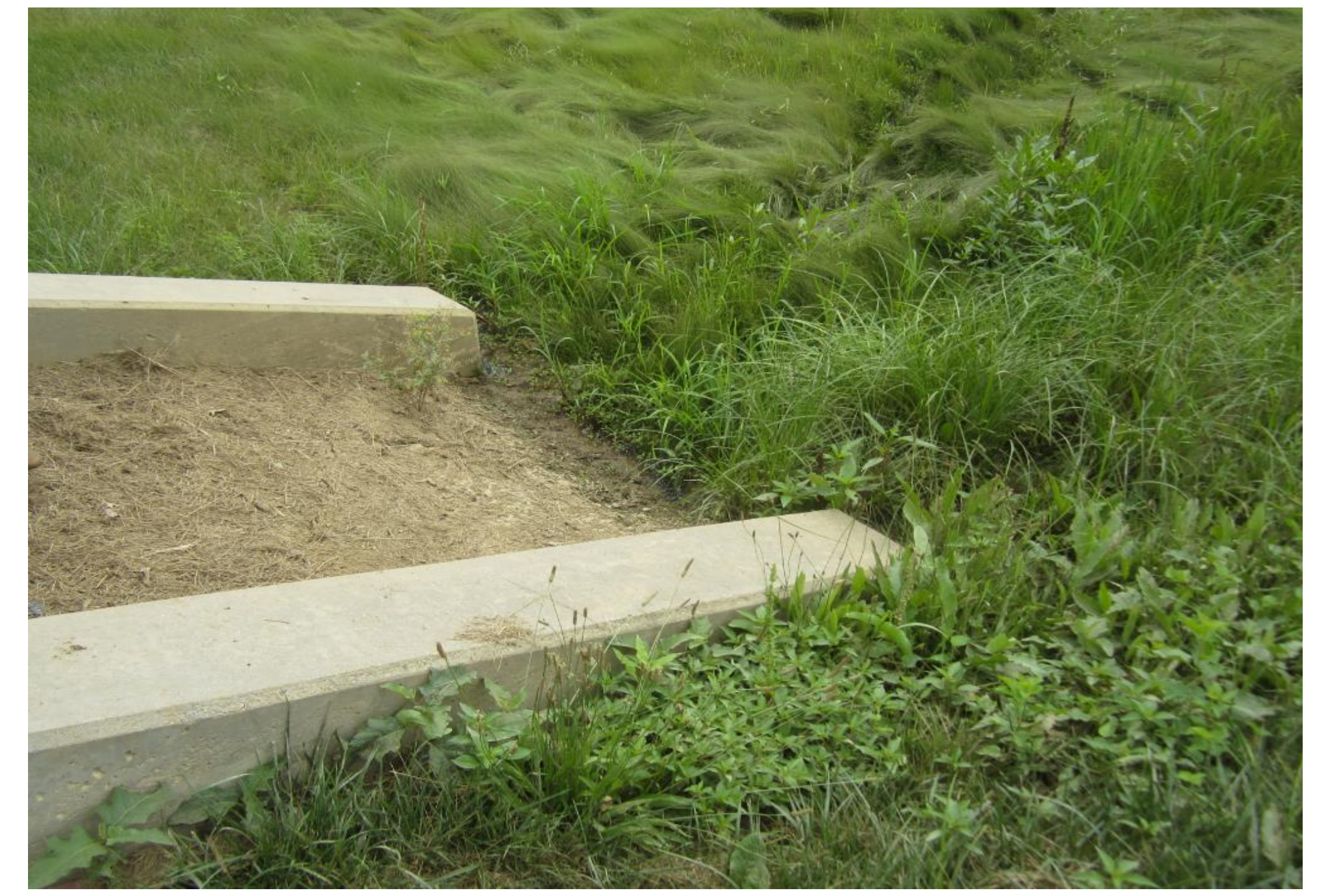
Grass clippings accumulated near outlet structure
