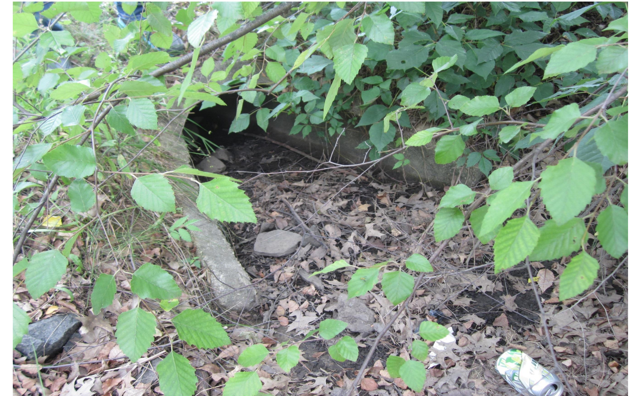
Debris, litter, and sediment accumulation near inlet
