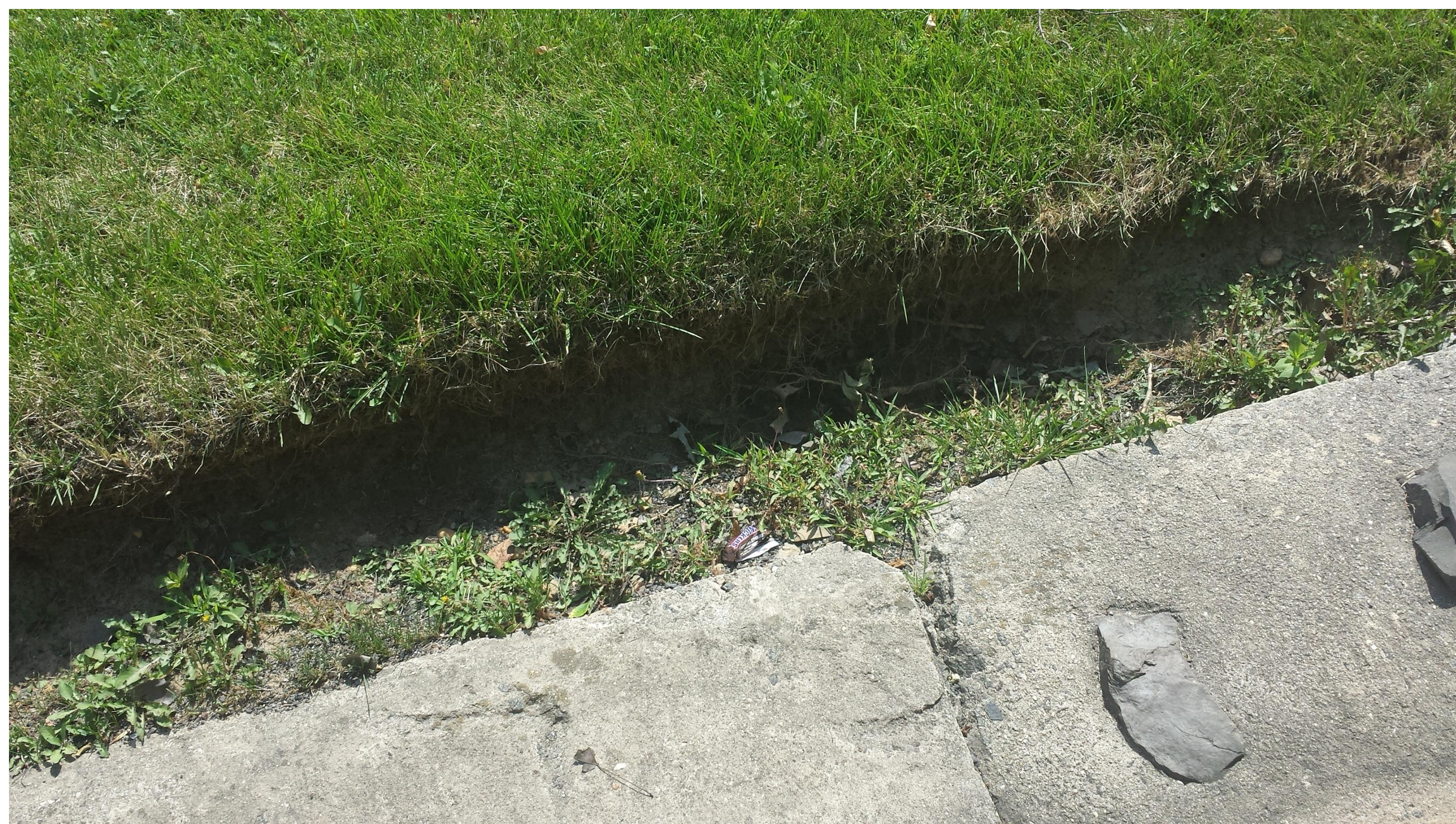
Erosion near inlet
