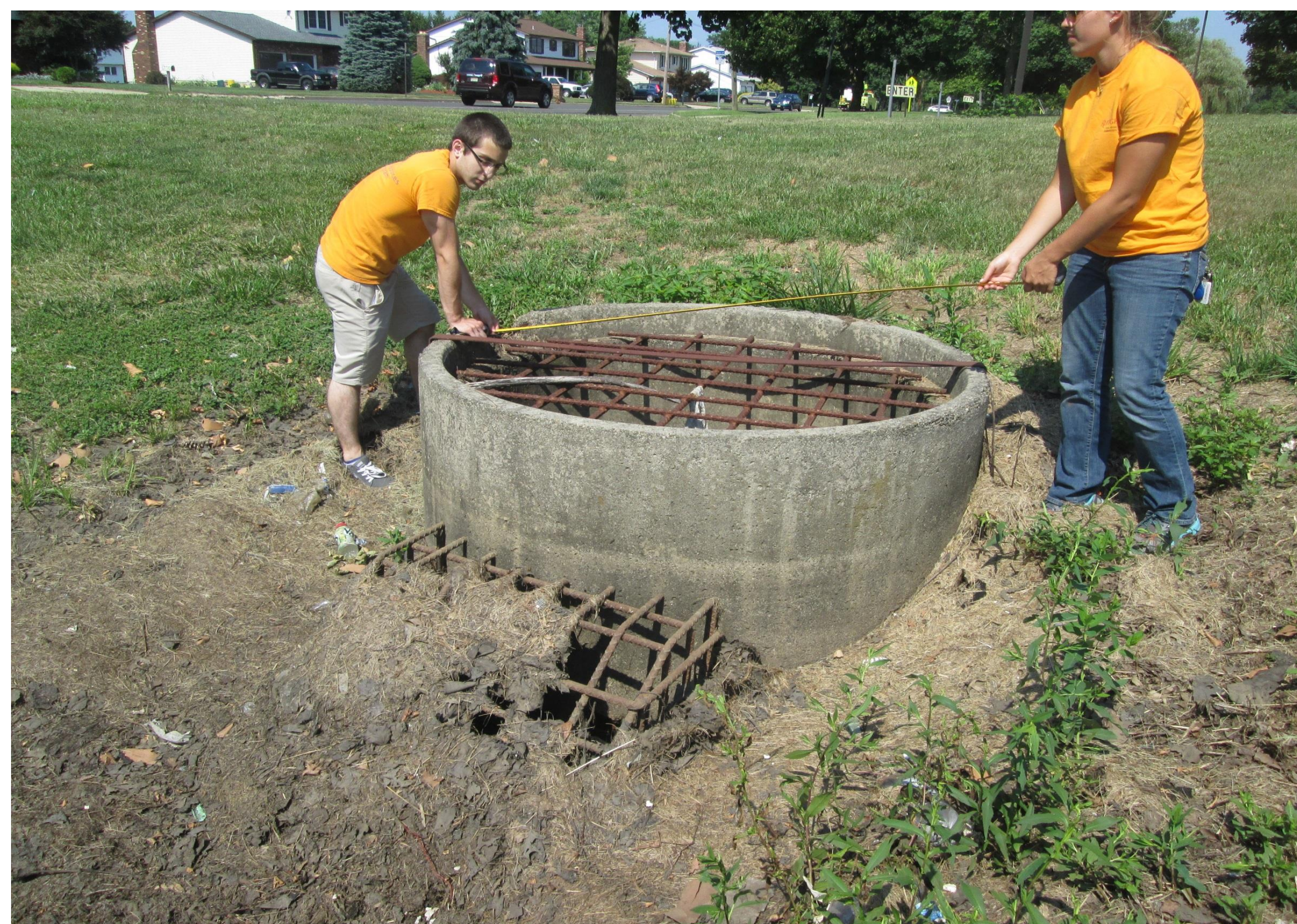
Degraded outlet structure
