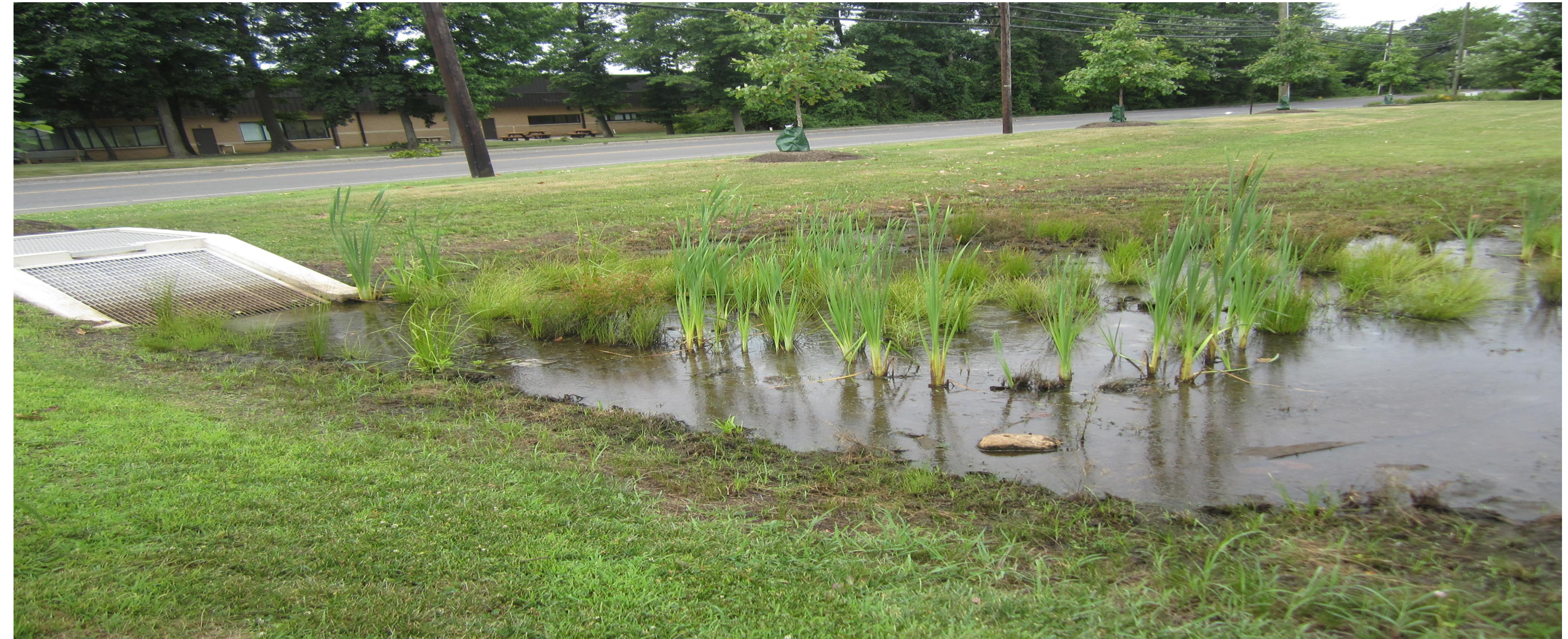
Standing water in basin bottom
