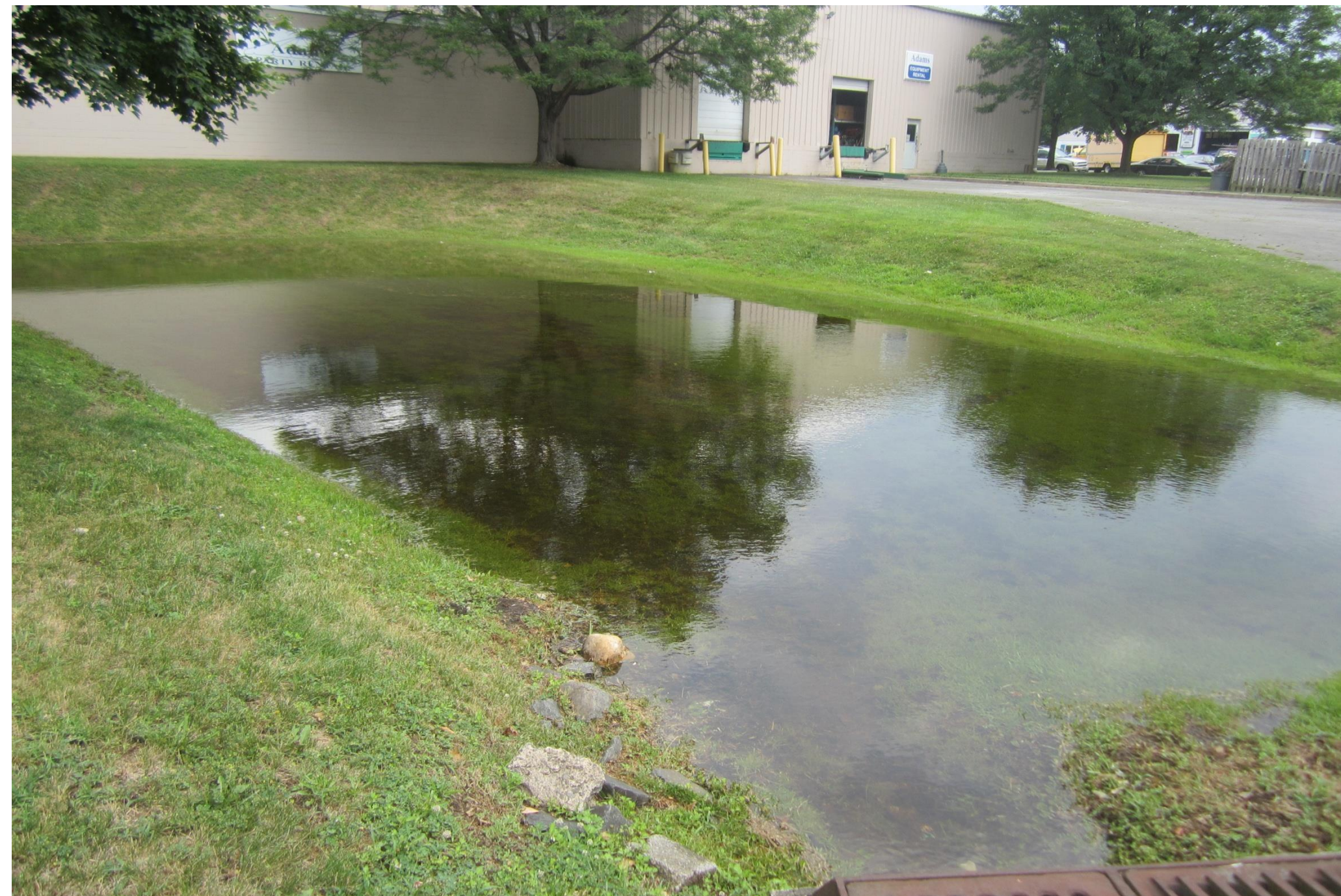
Severe ponding in basin
