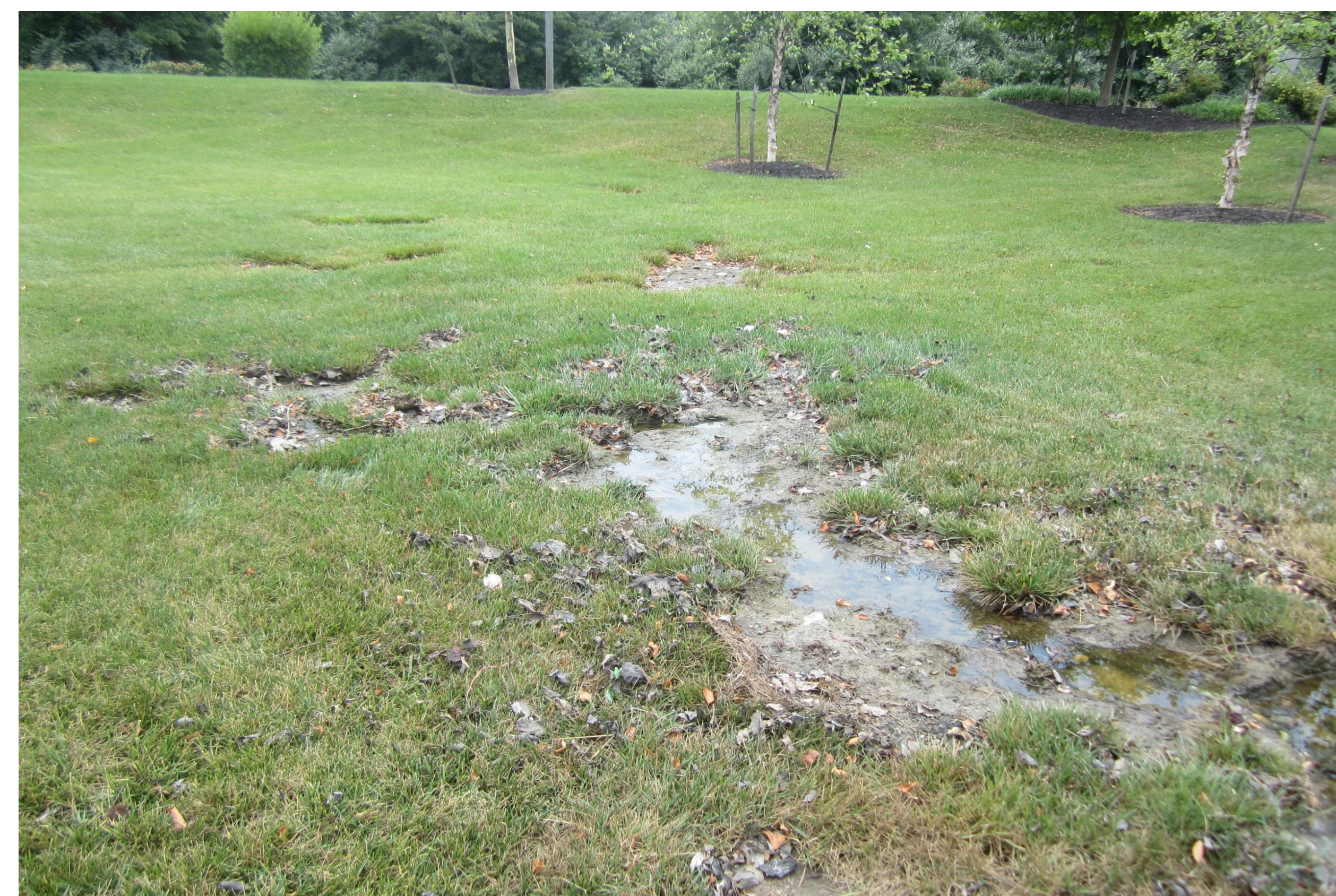
Exposed earth by inlet
