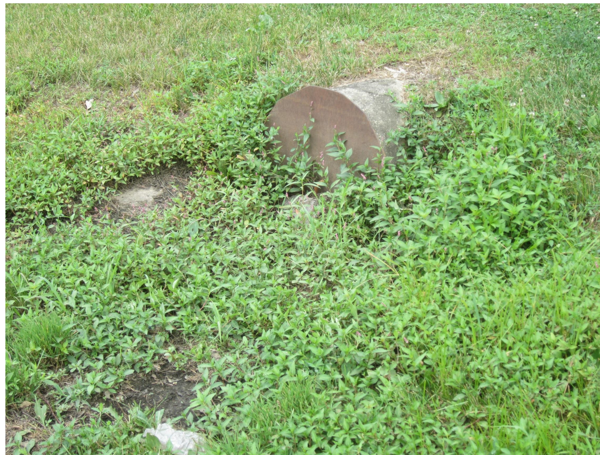
Invasive turf has accumulated in low flow channel
