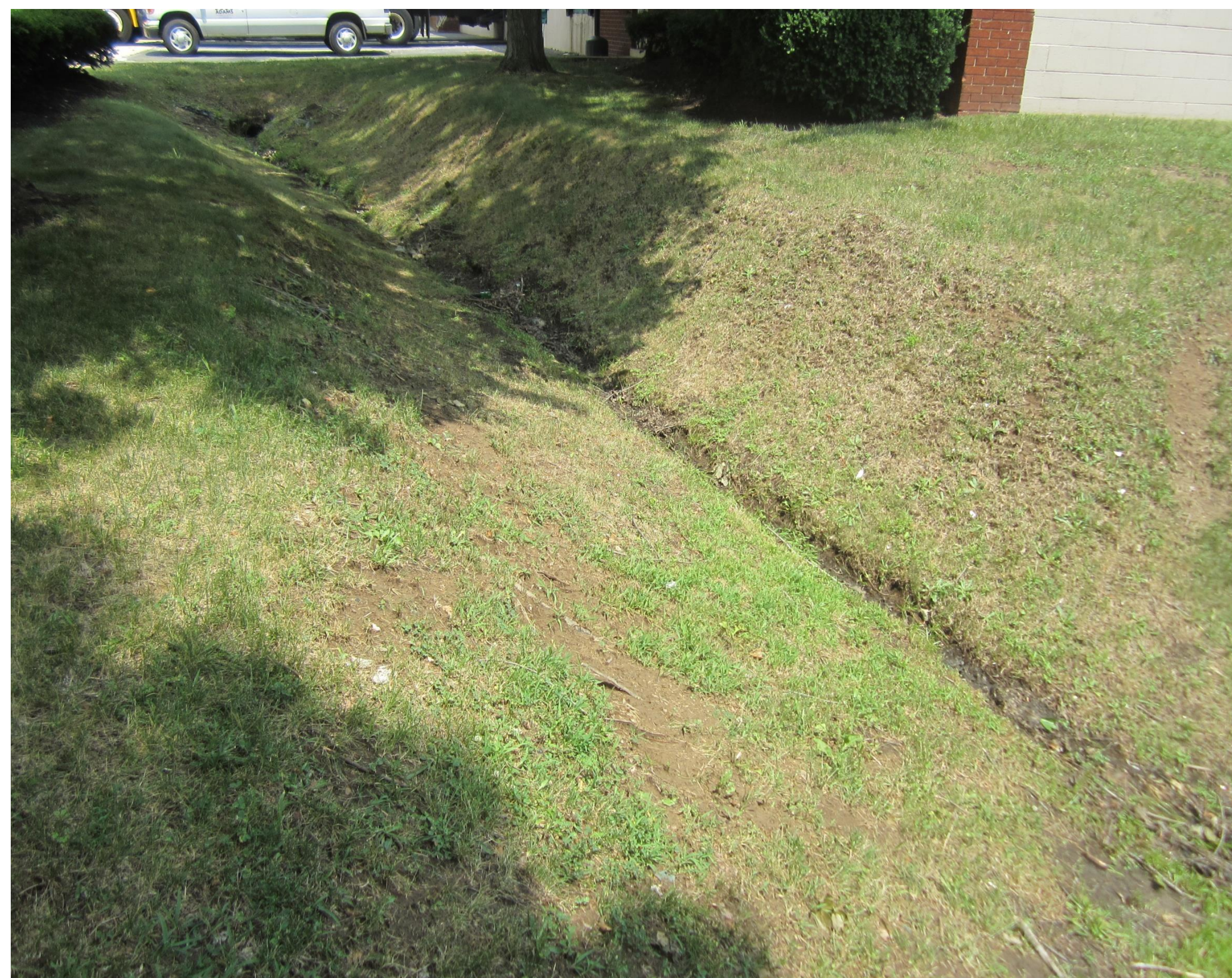
Eroded swale bottom
